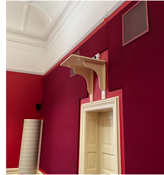
Council Chamber services are fed via air terminals providing pre-tempered air into the space via sidewall diffusers and dedicated ventilation pillars within corners of the room.
