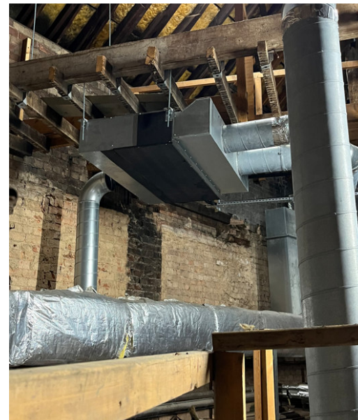
Ducted heating and cooling units to Victoria rooms within loft space, provided by fresh air by local fans. Unit over bar space.
