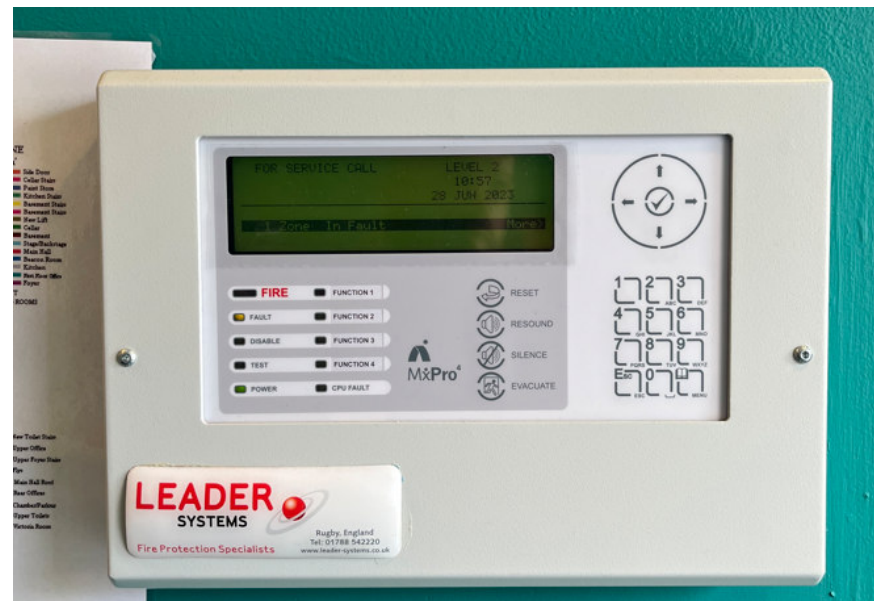
Fire Alarm panel in entrance lobby to Town Hall.
