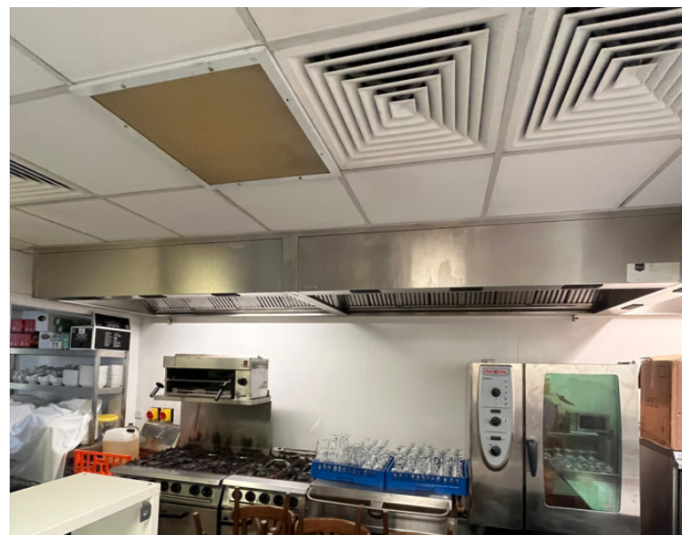
Kitchen Ventilation includes both 4 way blow grilles within ceiling and 2No. ventilation canopies over cooking equipment.
